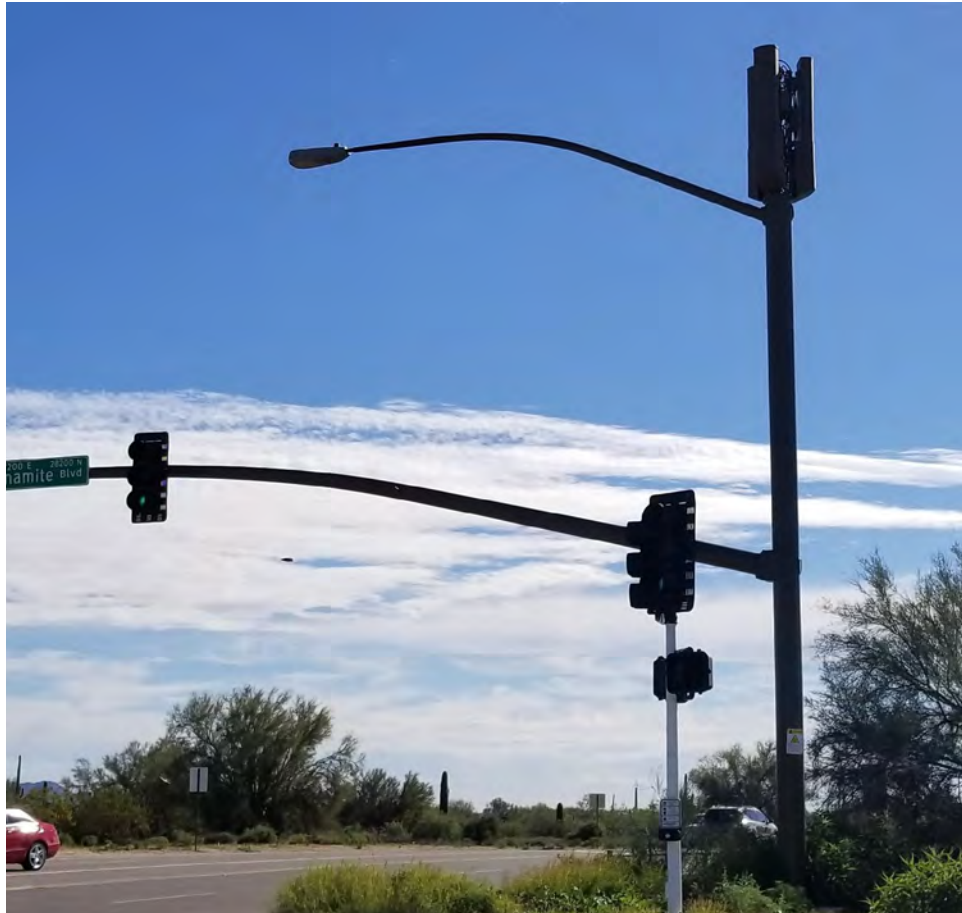
Small Cell Installation Nationwide
