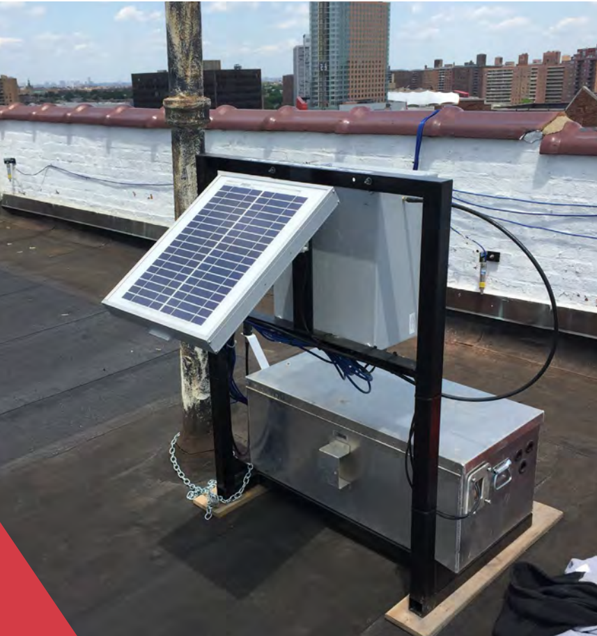
NYCDDC Tilt Monitoring, New York, NY
