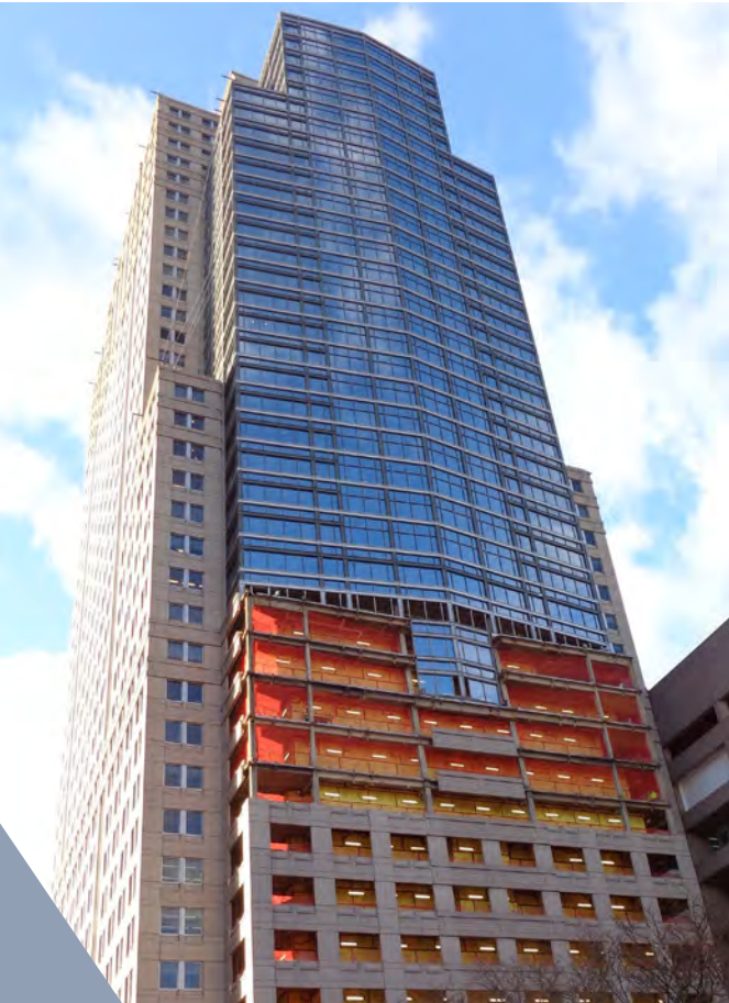
CitiGroup iDAS Installation, New York, NY
