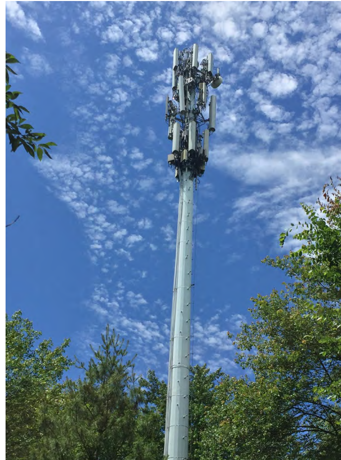
Telecommunication Structures Nationwide
