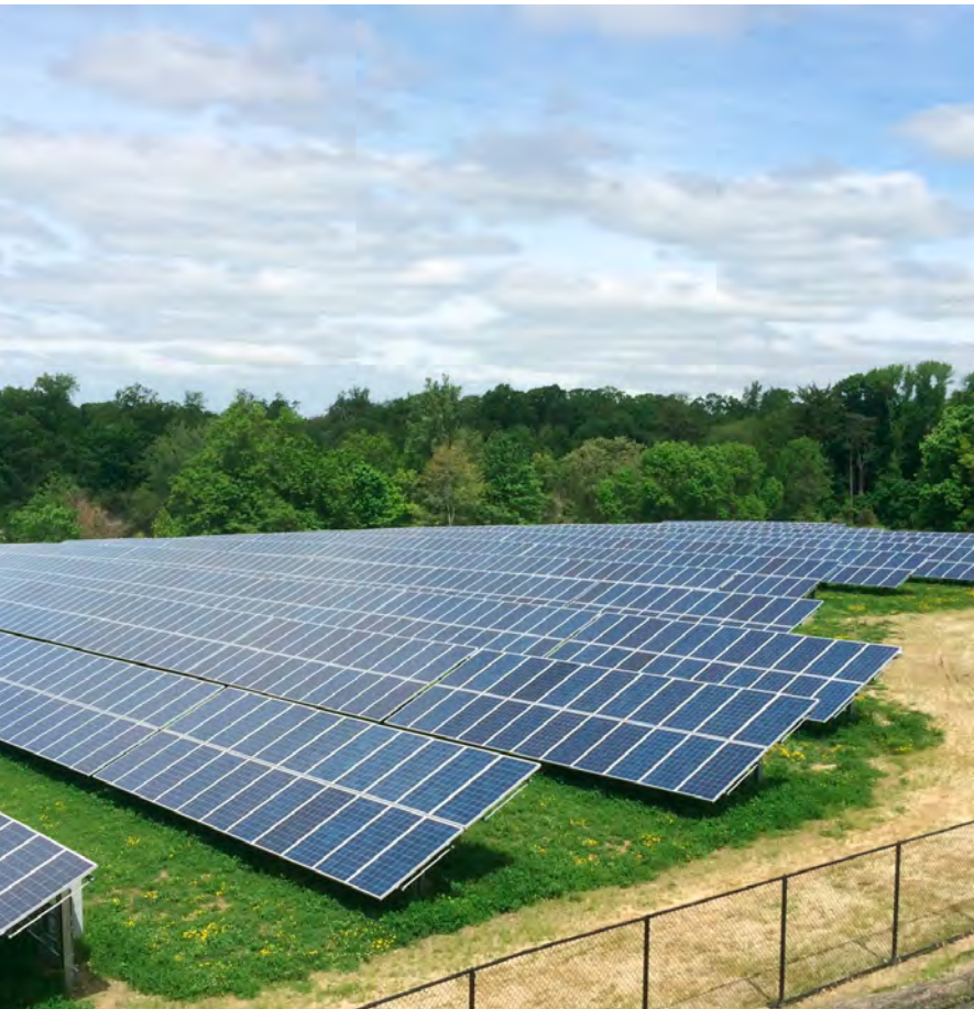
Morgan Stanley Phoenix Solar Array Installation, Westchester County, NY
