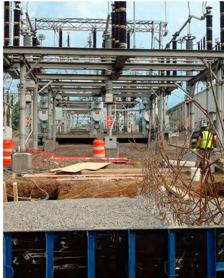
Consolidated Edison Sprainbrook Substation Yonkers, NY
